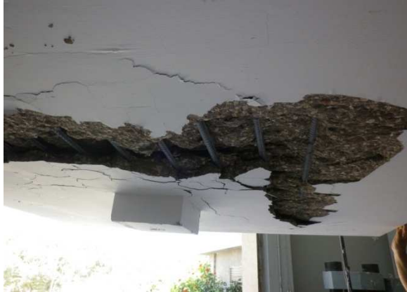
Figure 9: Mode of failure of PSW8-8.
